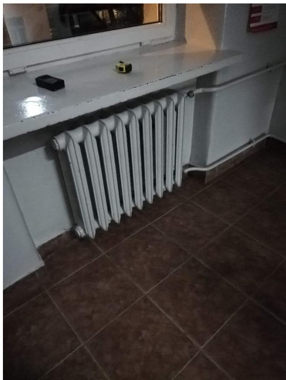
Parapet okienny instal CO
